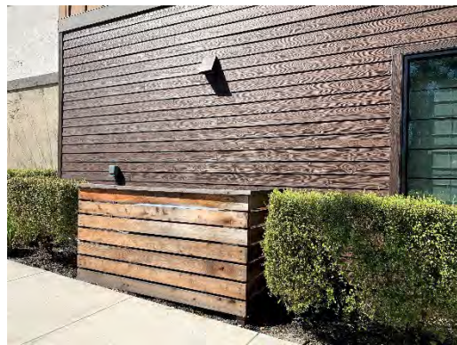
Screened mechanical equipment
