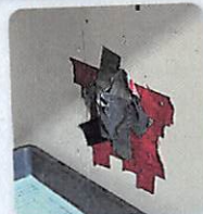
Aging city facilities need significant repairs or replacement to remain safe and functioning.
