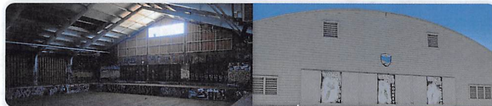
Recreation and aquatics facilities inherited from Fort Ord must be upgraded or demolished
