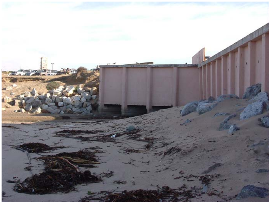
Figure 20: North side of the Monterey Beach Hotel. Rip-rap covered with sand. (Gref, 2004)
