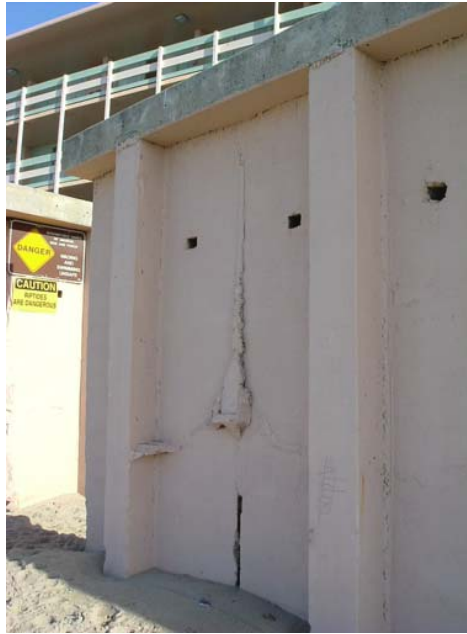
Figure 21: Part of cracked wall of the Monterey Bay Hotel. (Gref, 2004)
