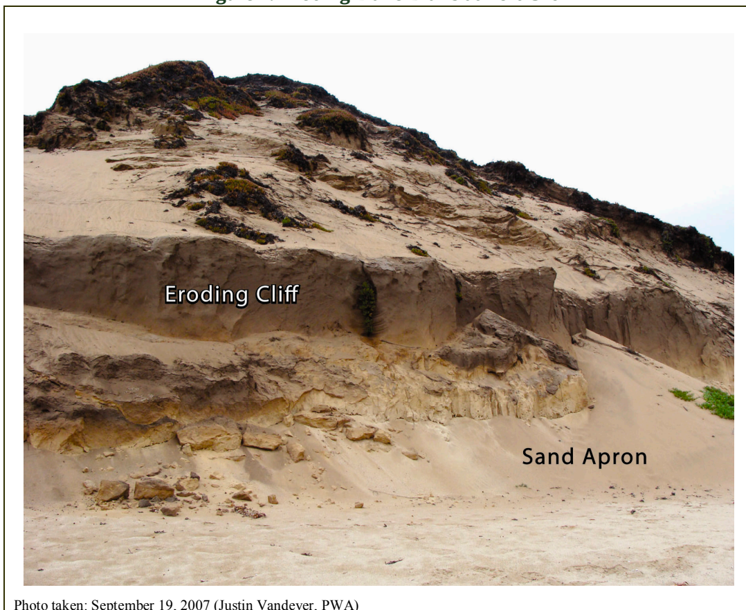
Figure 4. Eroding Dune Bluffs at Fort Ord
