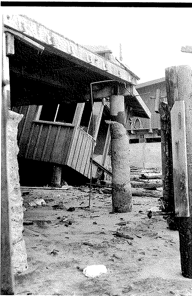
Figure 14. Scour of up to 2.5 meters of sand during the winter storms of 1983 led to loss of support for shallow pilings and collapse of this home onto the beach.
